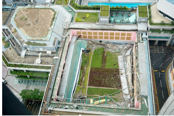
City University of Hong Kong Hu Fa Kuang Sports Centre roof collapses site
