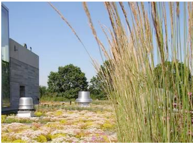
Semi-intensive green roof, Swarthmore College, PA, USA © greenroofservice.com
