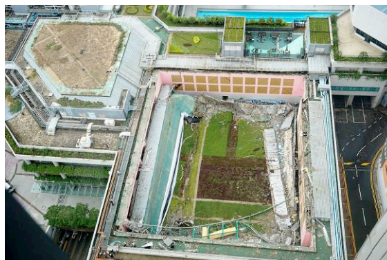
City University of Hong Kong Hu Fa Kuang Sports Centre roof collapses site
